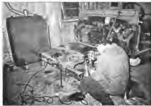
Metal surgery, slicing off the rotten front of the 109 with a cutting blade on a grinder, much better than using the gas axe.
